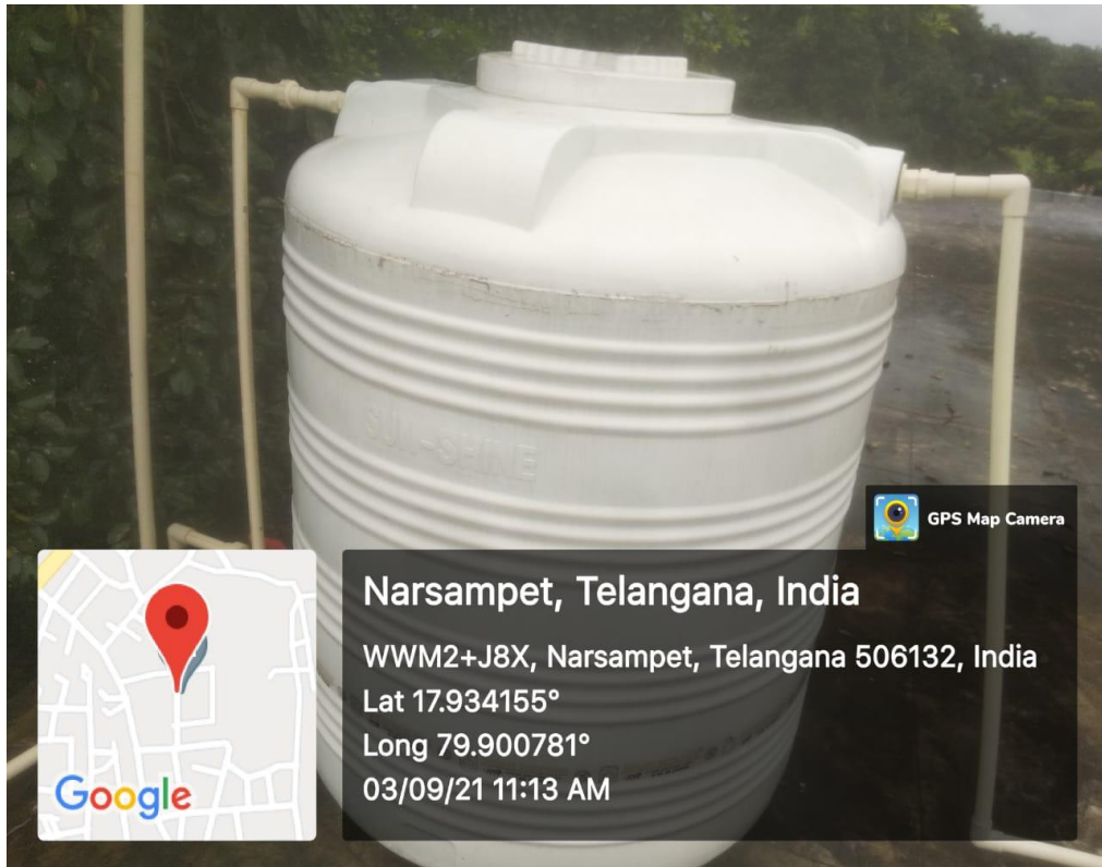
Water Distribution System in the College Campus
