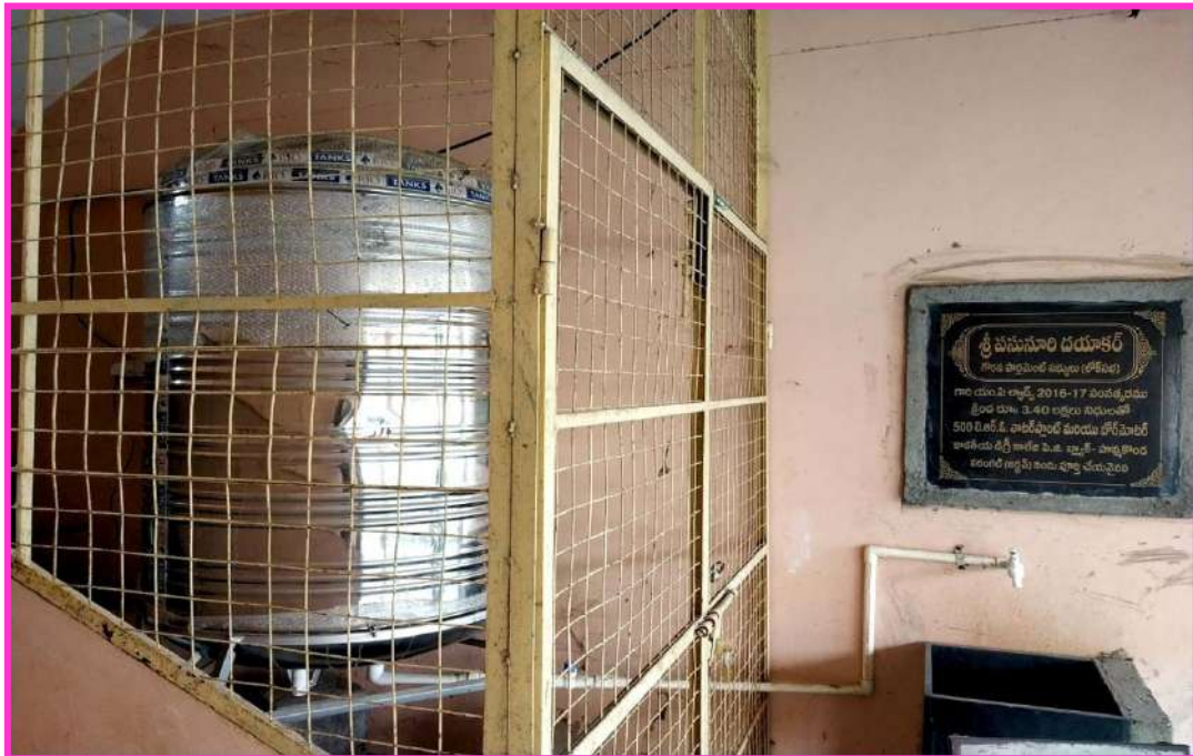
WATER PLANT -2 AT LIBRARY 2018-19
