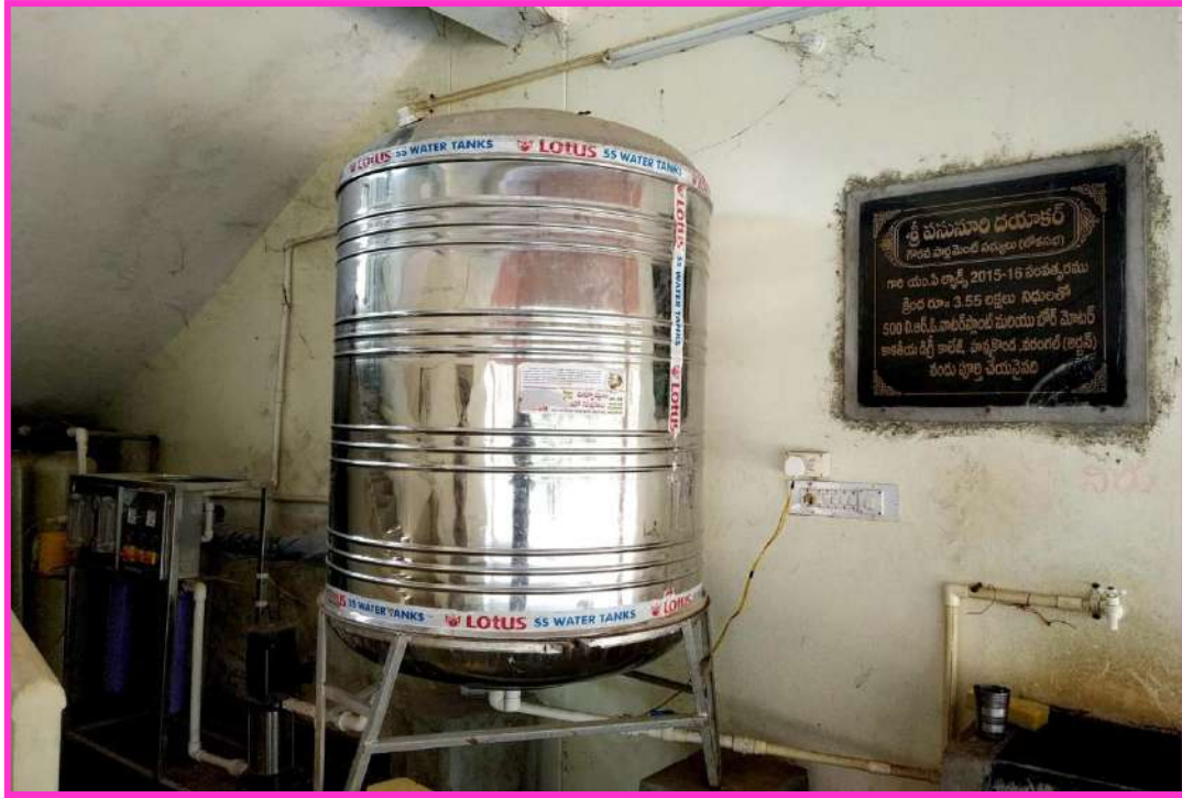
WATER PLANT -1 AT RUSA BLOCK 2018-19
